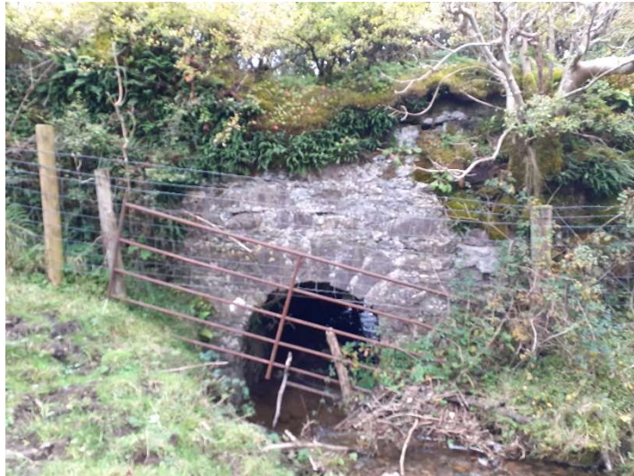
Figure 6 - Fragile bridge crossing within local secondary road L62031
